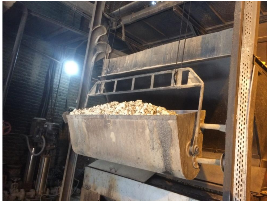
Figure 3: Feeding mechanism of a reciprocating grate biomass boiler (feeding corn cob)
