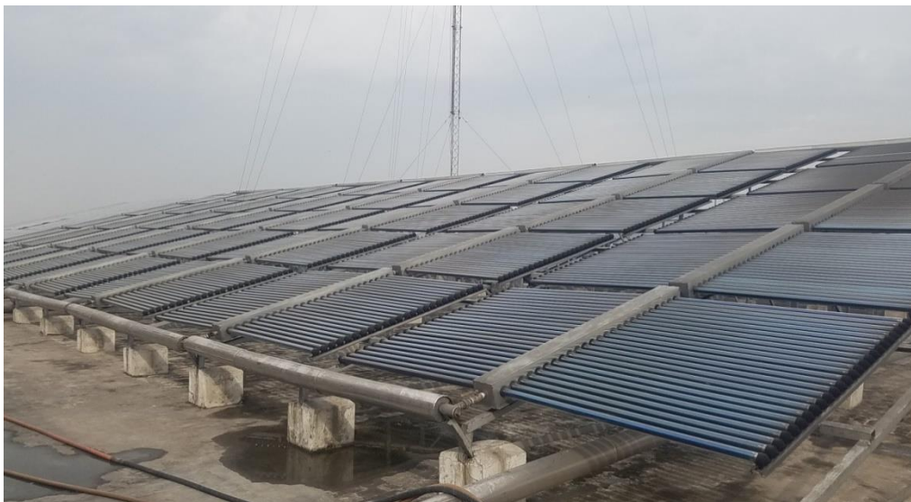
Figure 8: Solar water heater installed at a roof-top in Pakistan
