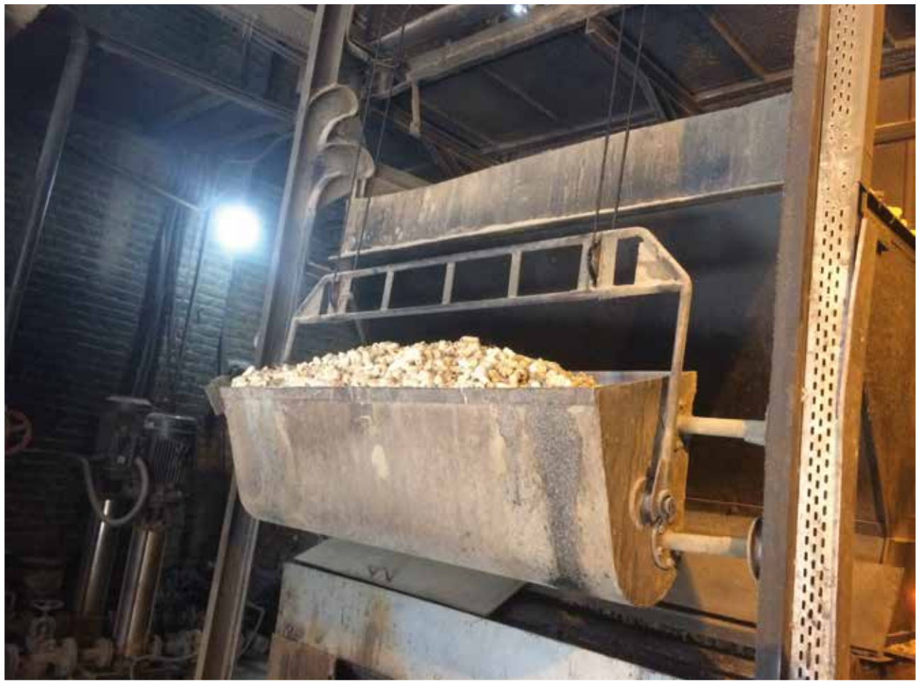
Figure 3: Feeding mechanism of a travelling grate bio-mass boiler (feeding corn cob)
