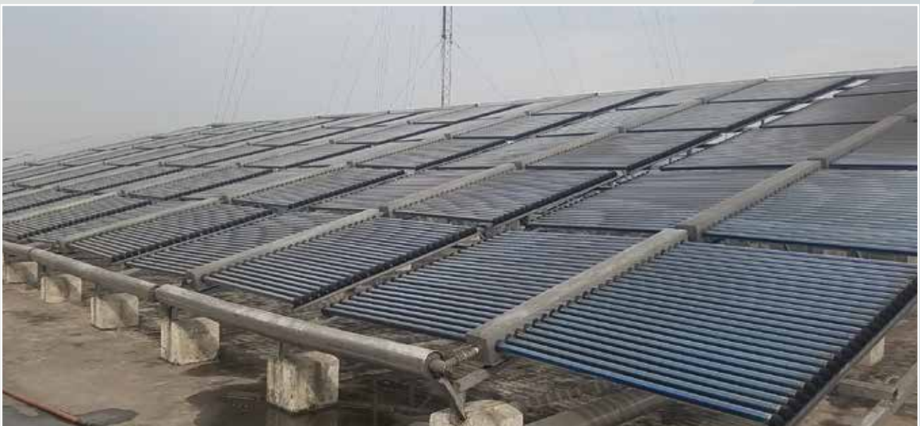
Figure 9: Solar water heater installed at a roof-top in Pakistan
