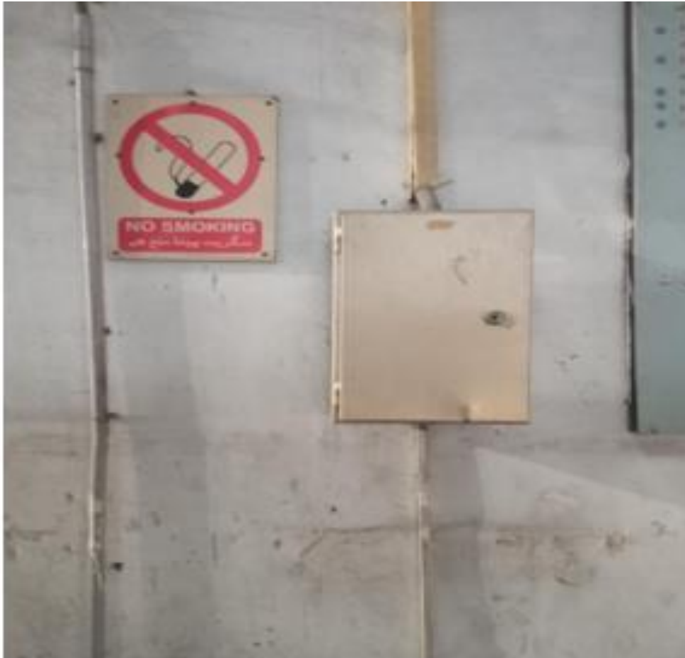
Absence of electric hazard symbols from DB board
