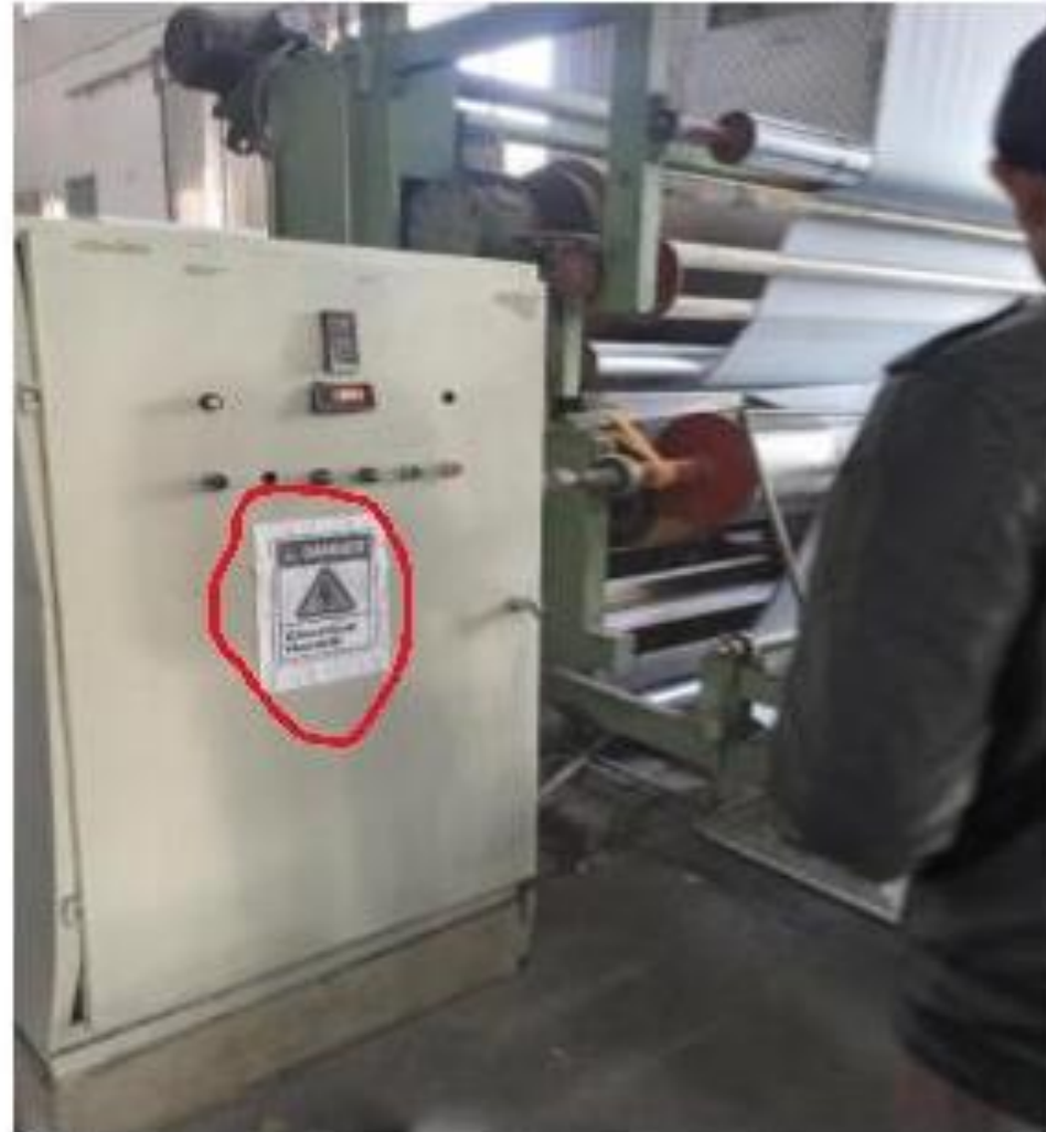
Implementation of electric hazard symbols
