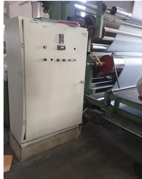
Absence of electric hazard symbols from DB board
