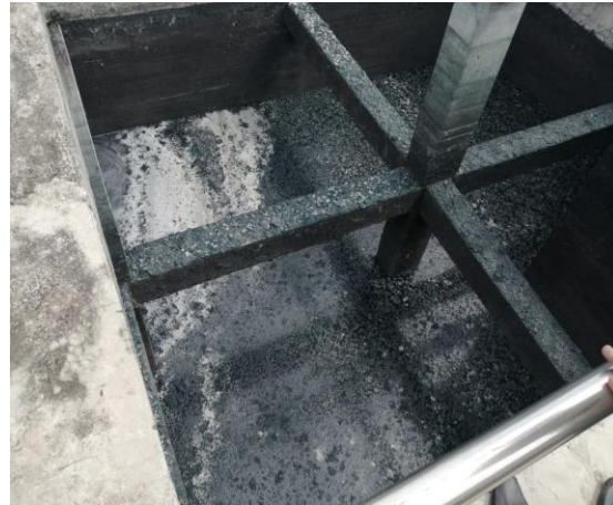
Sludge collection tanks
