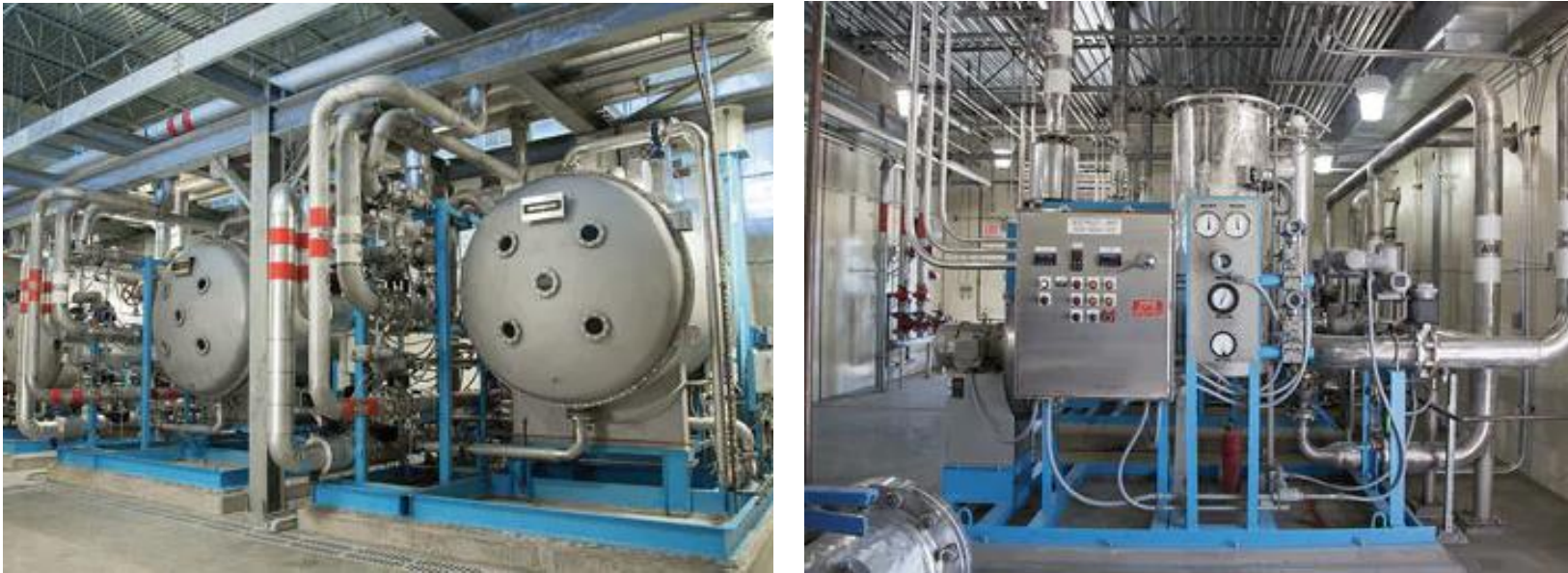
Ozonator (at Wylie Water Treatment Plant, North Texas)
