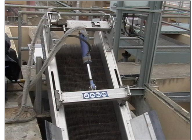
Mechanically cleaned screen
