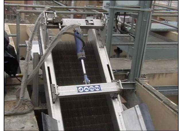
Mechanically cleaned screen
