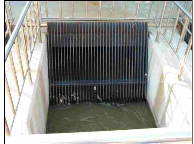
Manually cleaned screen
