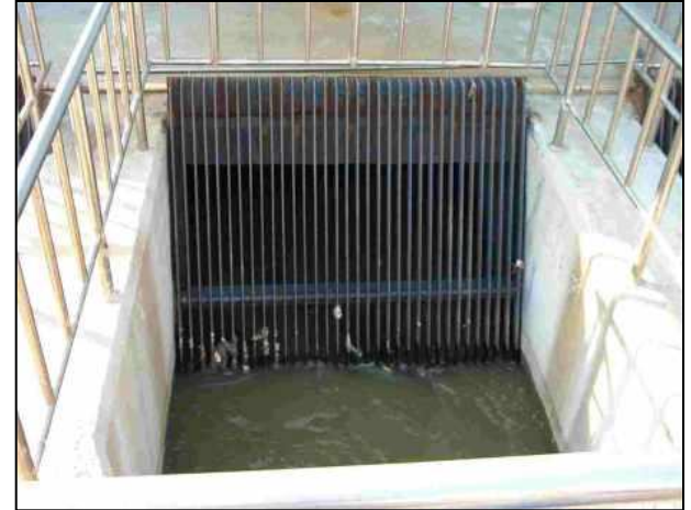
Manually cleaned screen
