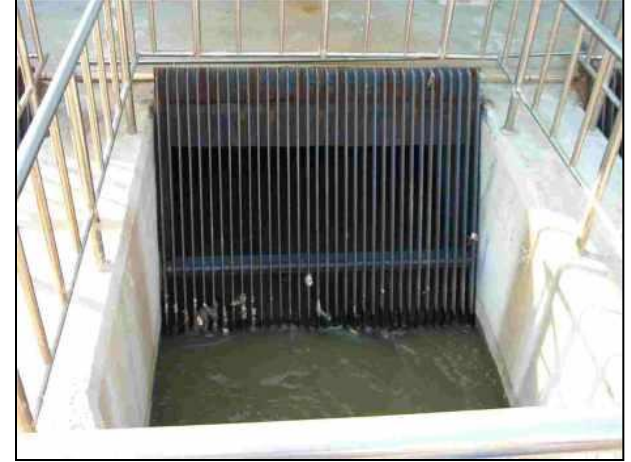
Manually cleaned screen
