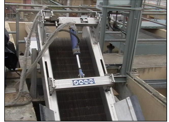
Mechanically cleaned screen
