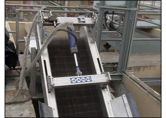
Mechanically cleaned screen
