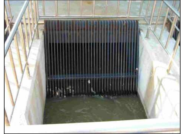
Manually cleaned screen
