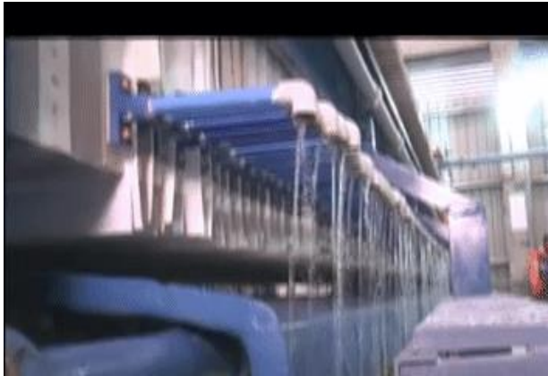
At beginning of cycle, filtrate flow even and high
