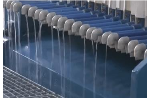
At end of filtration, flow slowing down to trickle, indicating filtration cycle getting completed
