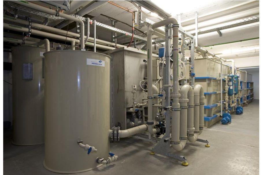
AOP system by Enviro Chemie
