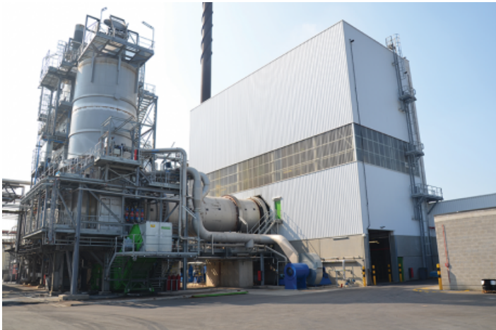
Figure 5 A industrial sludge incinerator in Antwerp, Belgium by Waterleau
