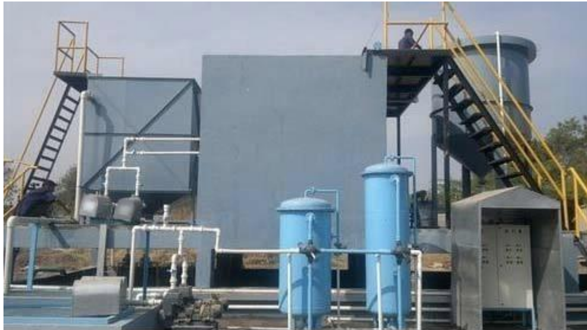
Fenton treatment unit by Xh2o Solutions Pvt. Ltd
