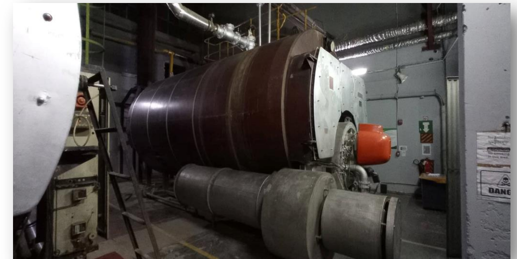
Gas boiler. Copyright: Kazi Farhan Hossain Purba
