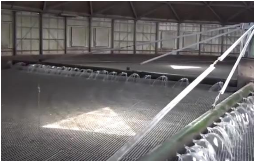
Trickling filter at Brunswick Sewer District
