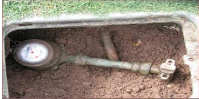
Pipe used to partially bypass water meter.
