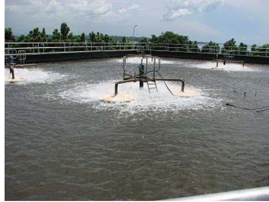
Figure 10 Wastewater treatment facility
