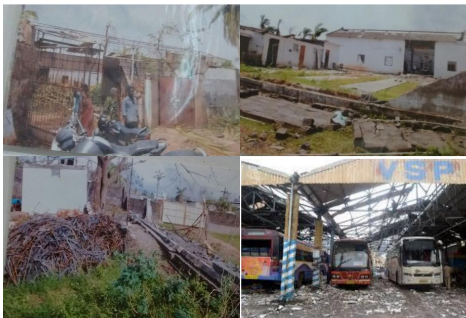
Figure 15: industries damaged due to severe cyclone –Hudhud
