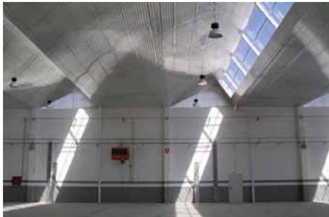
Image no. 3-20: Examples of Roof lights [Source: Murty & Manyam Architects and Engineers Ltd.]
