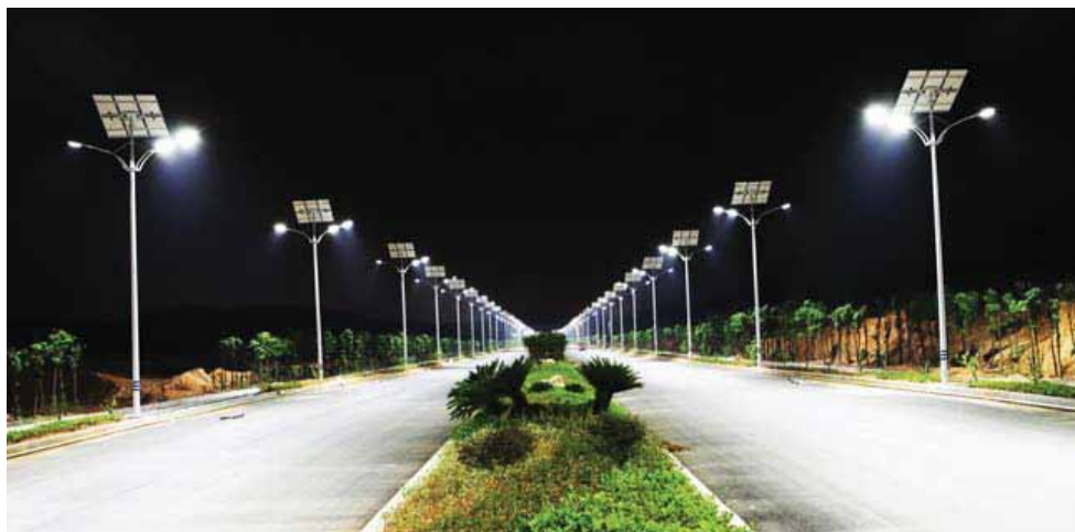
Image no. 3-23: Example of Solar powered LED Street lights
