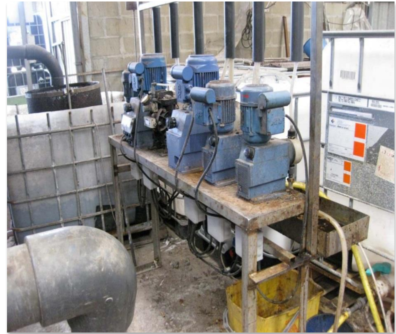
Inline pH controlsystem dosing pumps with PLC contolled system
