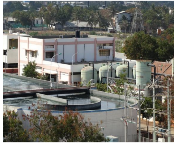
Biological Oxidation Tank
