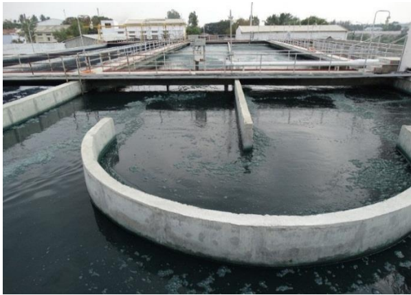
Biological Oxidation Tank
