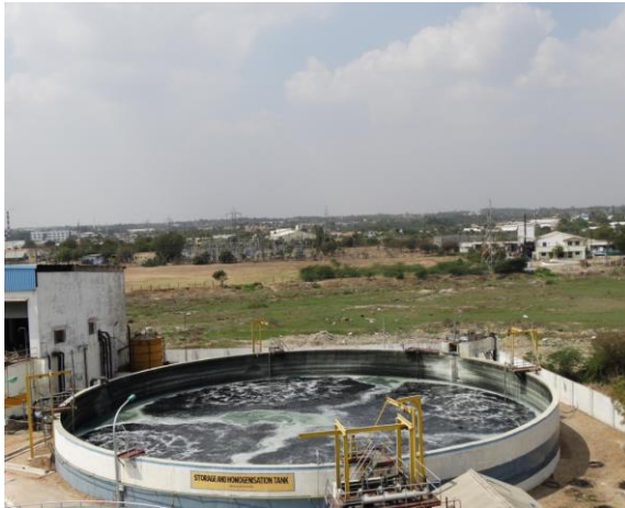
Storage and Homogenisation Tank
