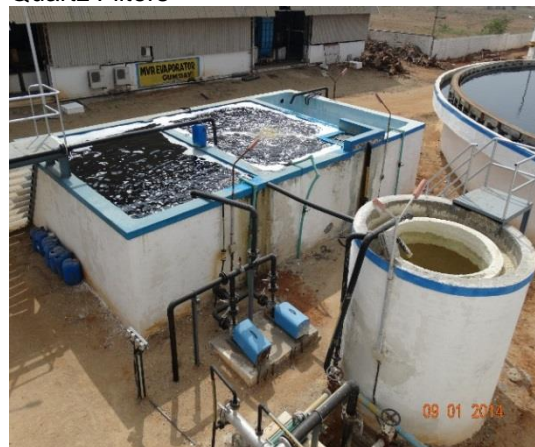
Reactor Clarifier System
