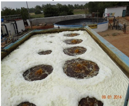
Brine Treatment System
