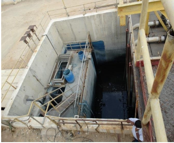
Lifting Pump station
