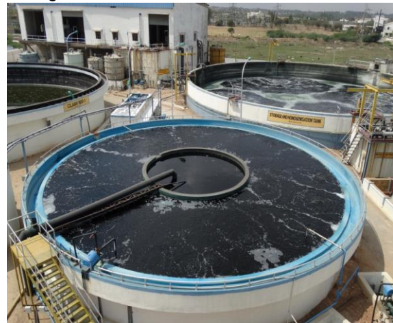
Colour Removal System
