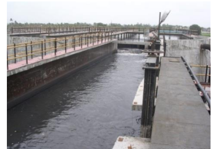
SBR Basin commissioning)
