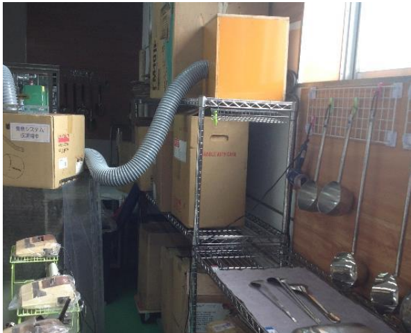
Dust collector in dyestuff weighing area
