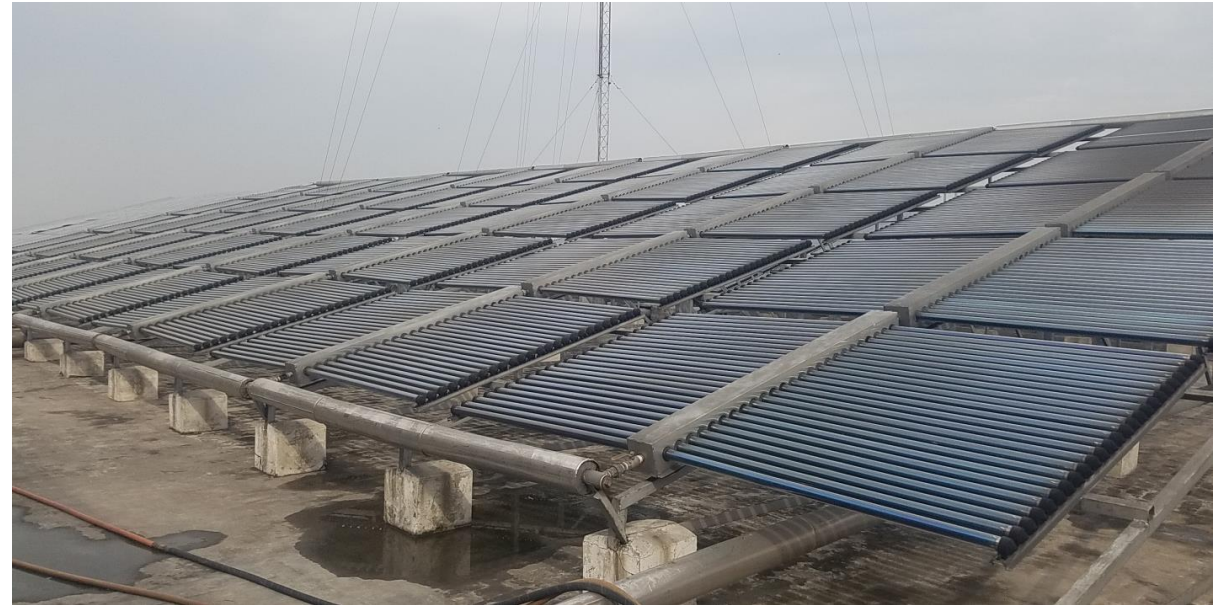
Solar Water Heating
